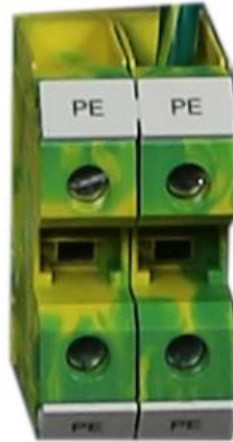
Figure 6: Ground Bus Terminal Blocks
