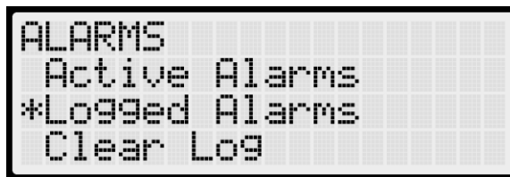
Figure 5: ALARMS Menu - Logged Alarms
