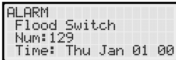
Figure 205: Alarm Part 1 of 2
