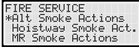
Figure 281: FIRE SERVICE Menu – Alt Smoke Actions, Hoistway Smoke Actions, MR Smoke Actions
